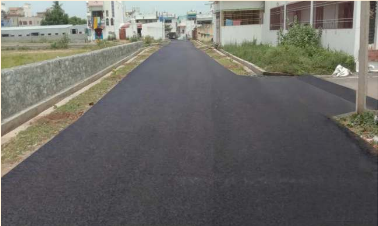
Providing BT Road at Rajarajan Nagar in Komarapalayam Municipality Scheme: Kalaingar Nagarpura Mempoattu Thittam, Project Cost: Rs.2.02 Crore.
