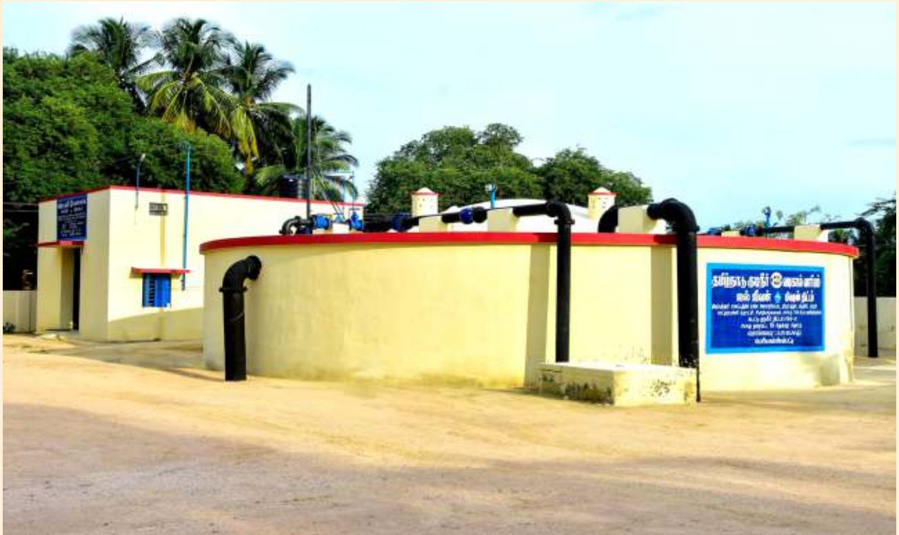
CWSS to 759 rural habitations in Jolarpet, Kandhili, Tiruppathur and Natrampalli unions in Tiruppathur district - 6.15 Lakh liter Capacity Sump at Periyakammiyampattu
