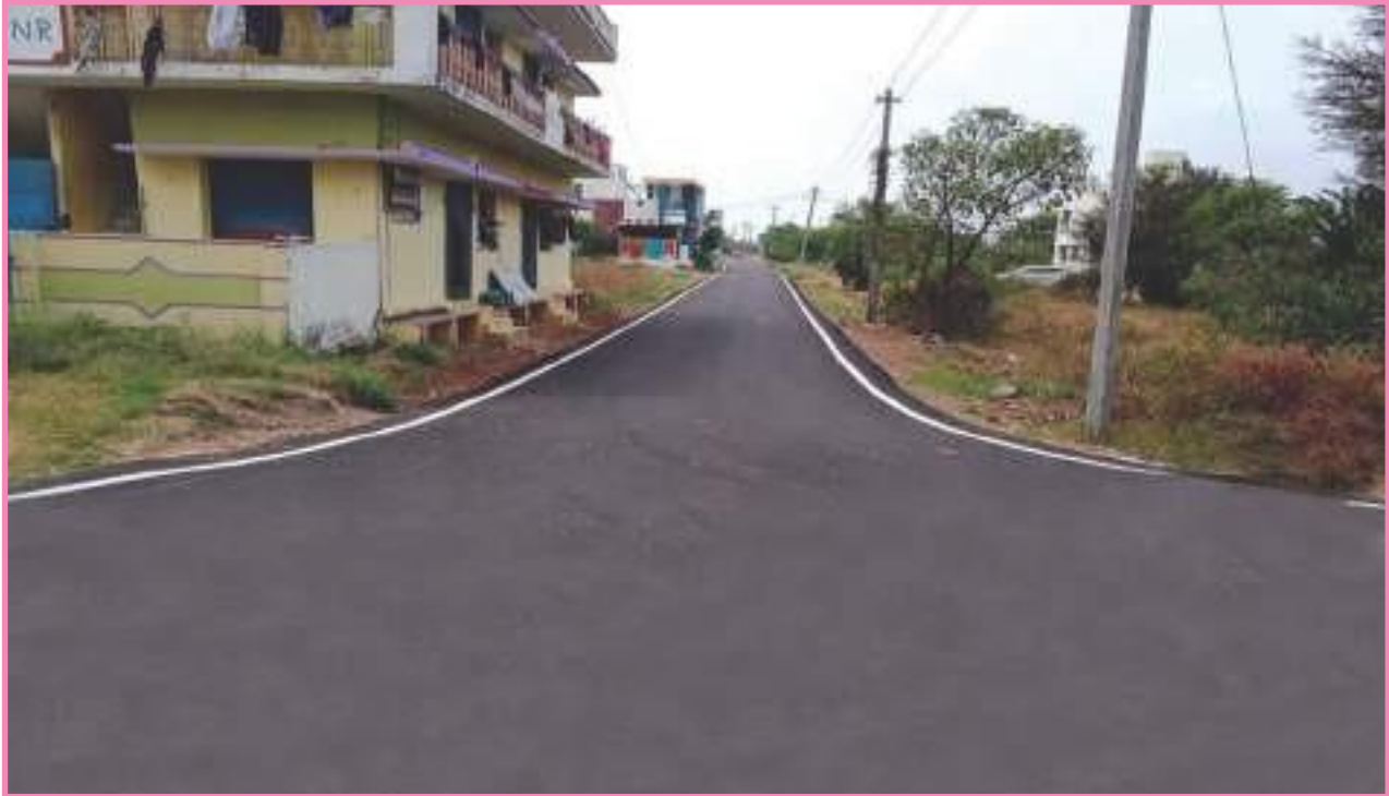
Development of BT road at Sungu Pettai in Perambalur municipality, Scheme : Kalaingar Nagarapura Mempattu Thittam; Project cost : Rs. 79.38 lakh
