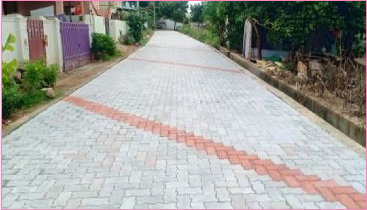
Construction of paver block road and stormwater drain at Sri Sampathkumar Nagar, Odayakulam town panchayat (Coimbatore district), Scheme : Kalaingar Nagarpura Mempattu Thittam; Project cost : Rs. 52.78 lakh
