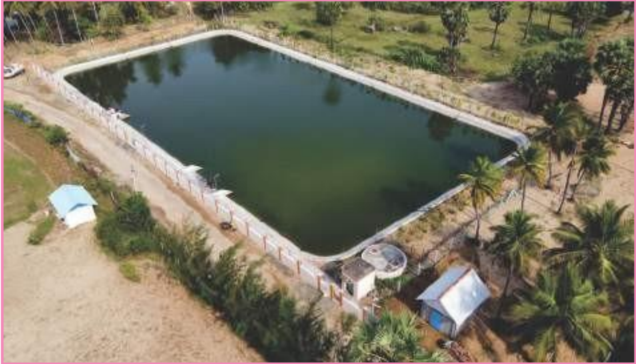
Rejuvenation of Vanadurgai Amman Kulam in Vedaranyam municipality (Nagapattinam district), Scheme : Kalaignar Nagarpura Mempattu Thittam; Project cost : Rs. 57.80 lakh
