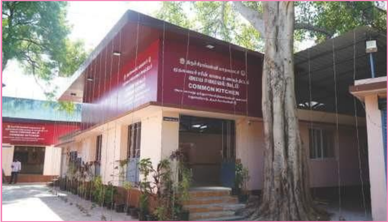
Construction of common kitchen in Tiruchirappalli corporation, Scheme : Chief Minister's Breakfast Scheme; Project cost : Rs. 1.29 crore
