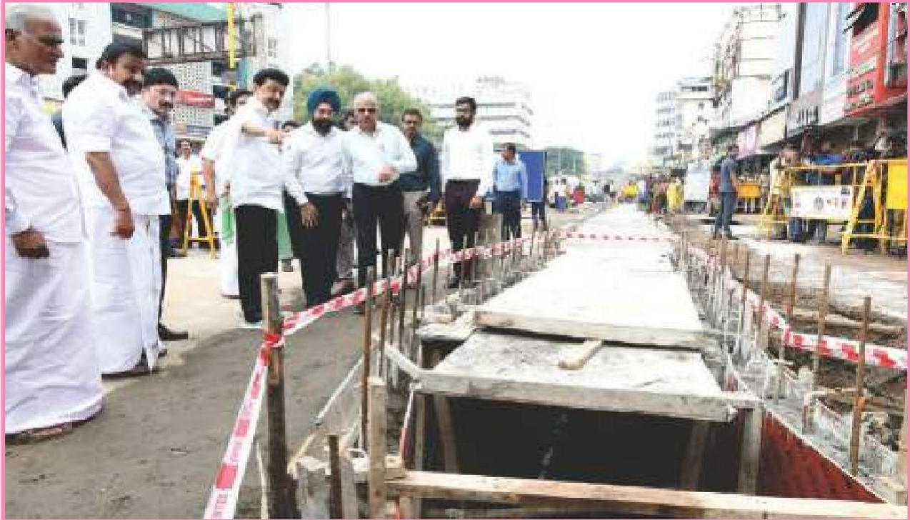
Honourable Chief Minister inspecting the stormwater drain work at Nethaji Subash Chandra Bose Road in Chennai city on 08.10.2022
